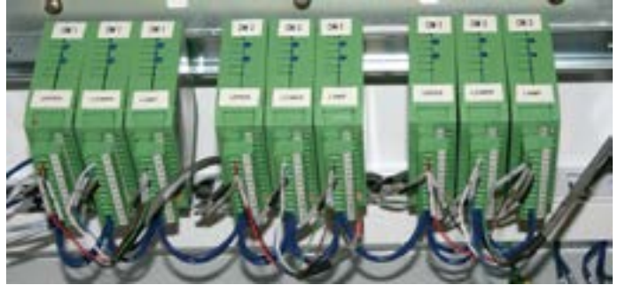
EIT DIN Rail units installed in cabinet to support multiple Compact Sensors used in production.
